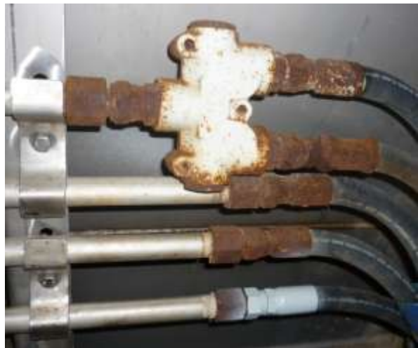
Fittings without shrink wrap when unit is not cleaned properly
